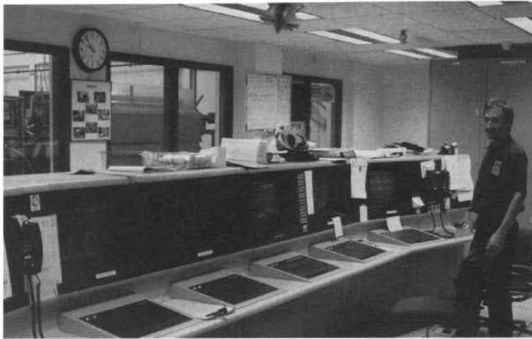
Control central for the MMSD facility.
