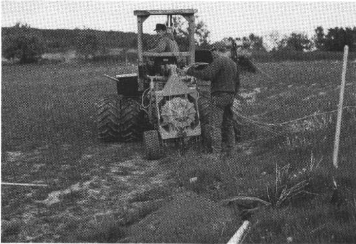
Midwest Irrigation pulled the main lines and control wires into the ground at the same time.
