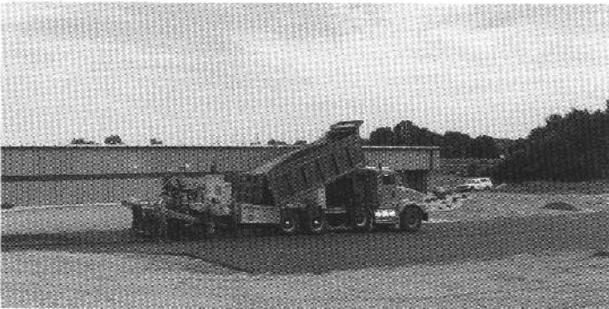
The finish layer of asphalt for the entry road and parking lot is being dragged down here.
