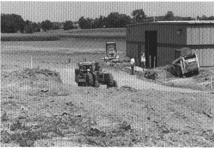
Stone wall construction and compaction of gravel base for the shop apron are taking place here on the west end of the building.
