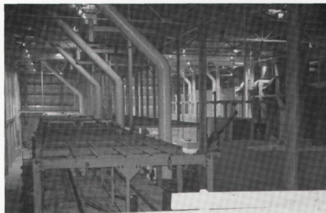
A view of a part of the painting addition now nearing completion.
