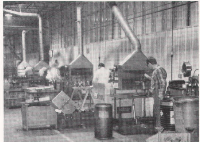
Welding fume collection system over small parts welding area.
