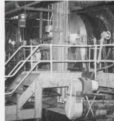
Jones Island Dryers 1981.
