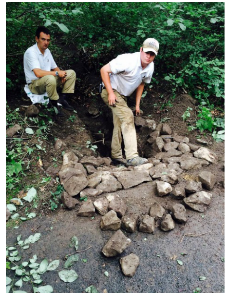
Nicholas Gmeinder and co-worker Carlton Henry fix a buried and clogged drainage pipe at Oakmont Country Club.
