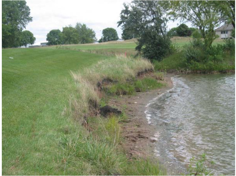
Typical pond erosion where the bank is being eroded away. Your options for repair may be limited depending on your pond permit.
