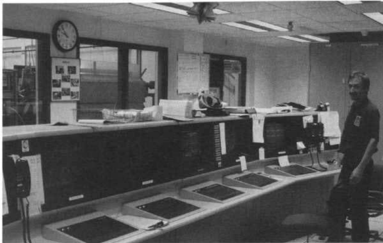
Control central for the MMSD facility.
