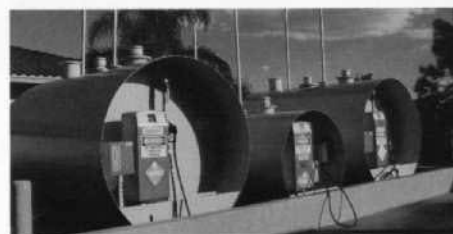
The turf tour visited Grand Cypress' shop, where we saw fuel storage and containment facilities second to none.
