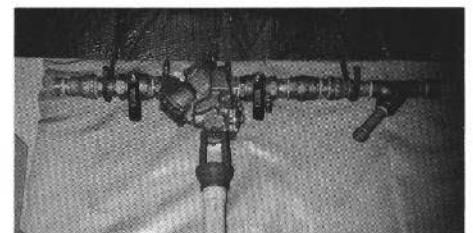
Reduced pressure principle backflow (RPPB) prevention device to be installed as our main fill source from our irrigation system.
