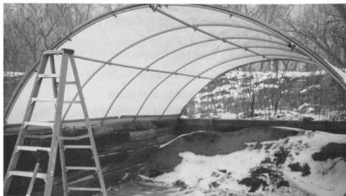
The front and back are left open. This allows the wind to blow through the structure
