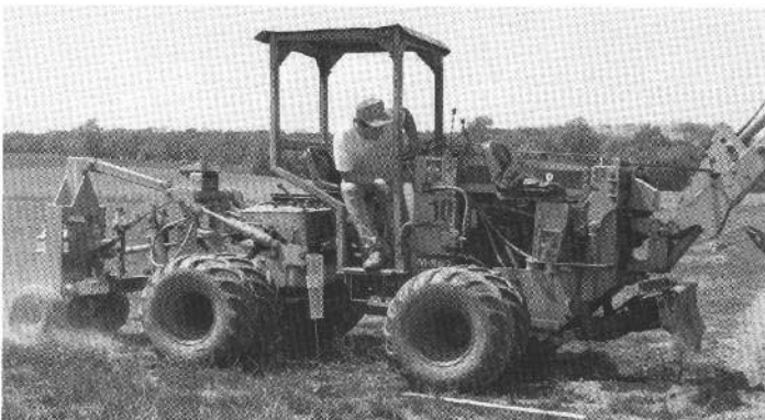
In this picture the plow is pulling poly pipe along the perimeter of a plot.
