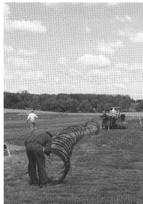
The irrigation system required thousands of feet of poly pipe.
