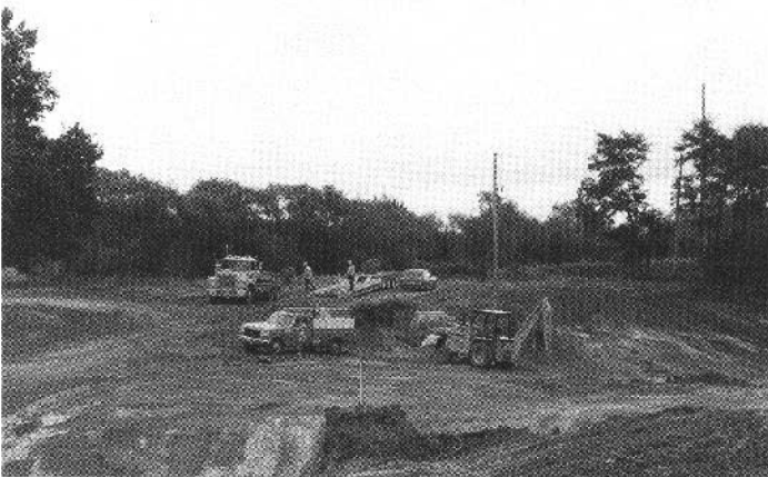
An underground fuel tank was removed "by the book, to the letter".
