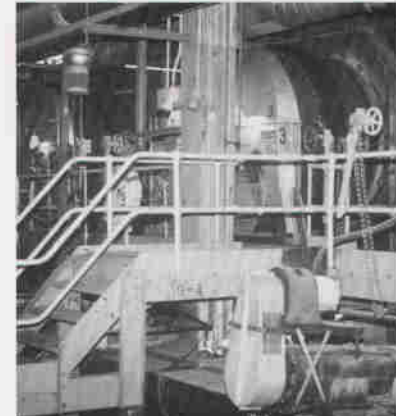
Jones Island Dryers 1981.
