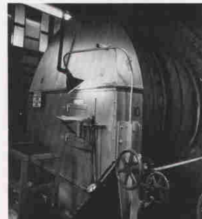
Jones Island Dryers.
