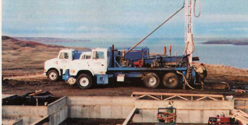
A well-drilling rig goes to work next to one of Sutton Bay's living quarters.
