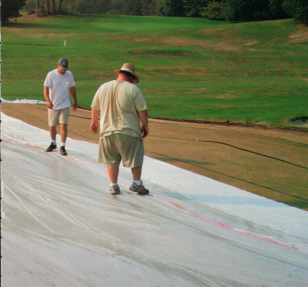
As workers at Gulph Mills GC prepare to use methyl bromide on the course's Donald Ross-designed greens, they tamp down tarps to keep the gas contained.
