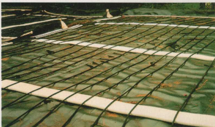
The small diameter pipes combine the subsurface irrigation and air delivery components of the Pennfield system. The white, flat pipes provide drainage and help recycle water from rainfall and irrigation cycles.
