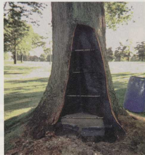
Once the rods were in place, a protective covering was used to line the inside of the tree.
