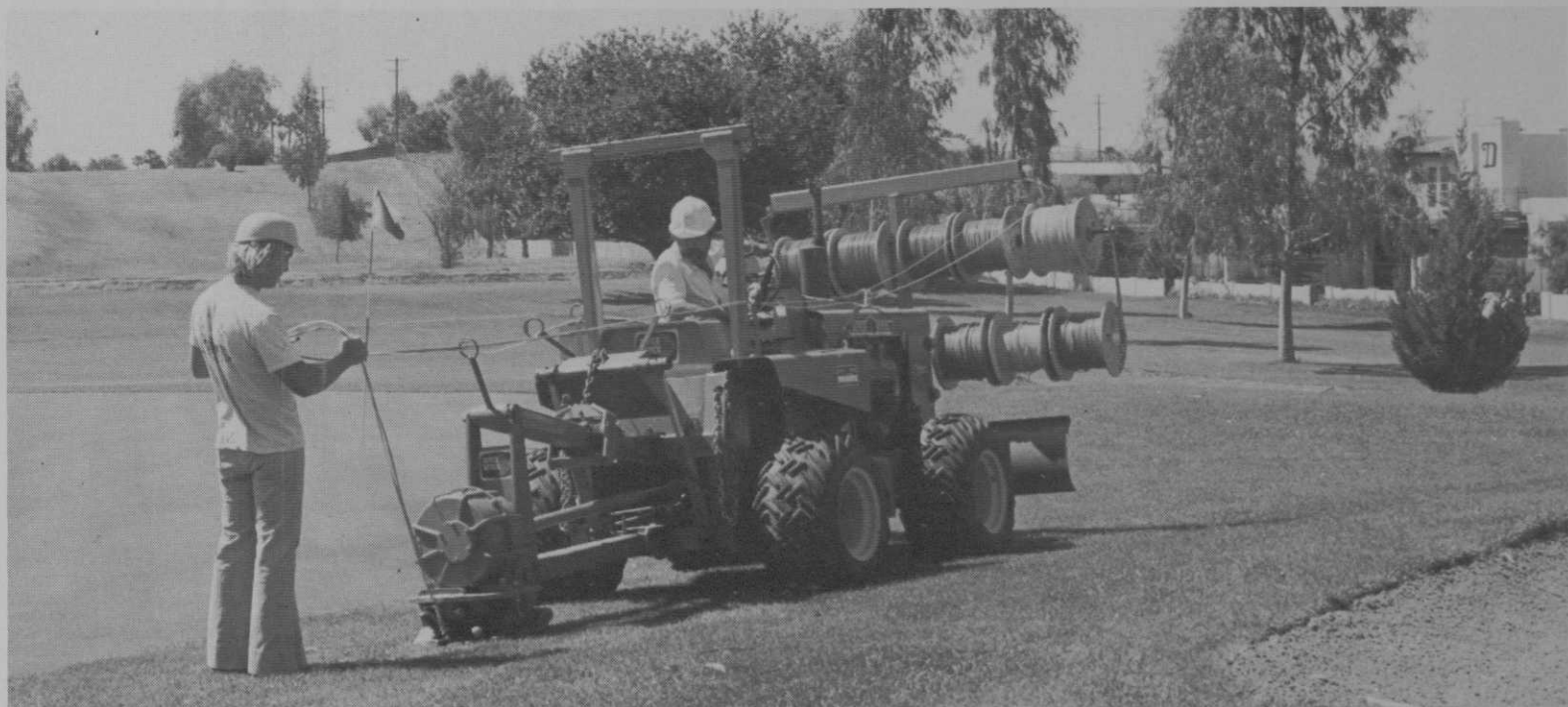
Vibratory plow installing irrigation system at Mesa (Ariz.) Country Club. Pipe and wire go in the ground at the same time.
