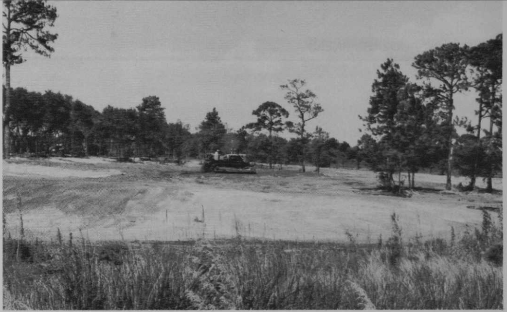
Construction of number 4 green on new executive-length Fairgreen Golf Course in New Smyrna Beach, Fla., designed by golf architect William W. Amick. During and before this stage especially close attention must be paid to the basics of turfgrass establishment.
