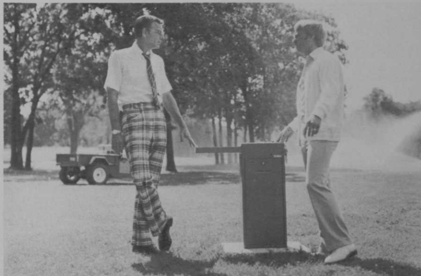
Director of Golf Jim Lucius and Superintendent Sonny Faust check one of the satellite controllers of the Southern Hills irrigation system.
