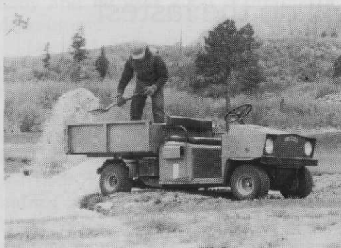
Broadmoor employees did supplemental jobs on course construction (such as filling traps with sand) to hold down labor costs.
