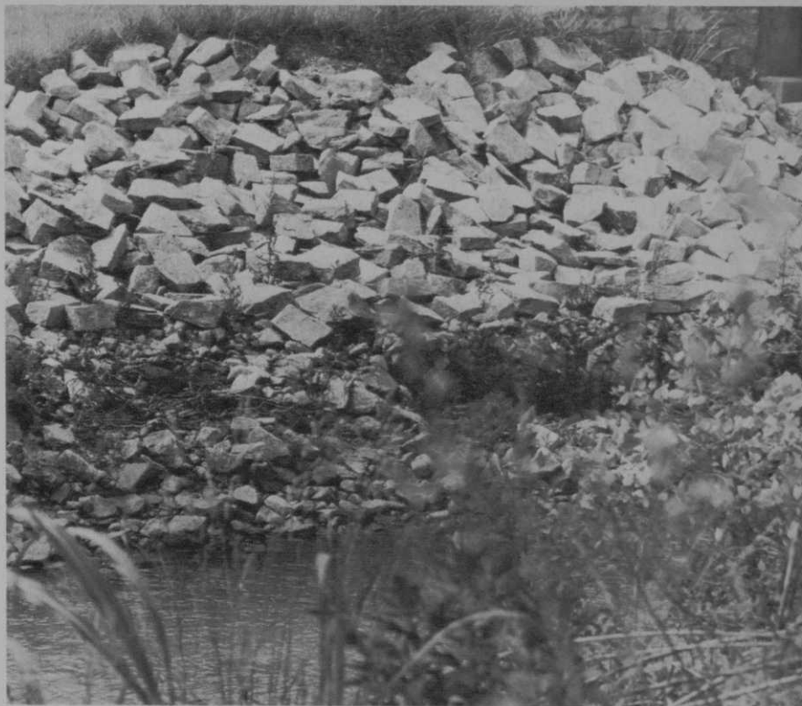
Rip rap and gabions line the banks of Snapfinger Creek in many places along the course to stabilize the banks and prevent erosion. Eventually the rocks will collect silt and support the growth of grass and small shrubs.
