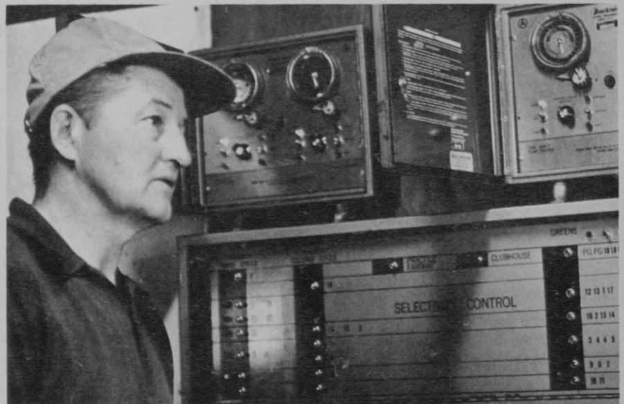
Coordinated operations are provided by custom-built control panel, located below central programmers in the main maintenance building at North Oaks.
