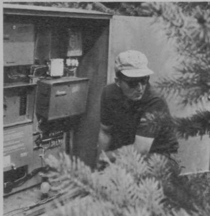
Dick Toupal at one field controller station.
