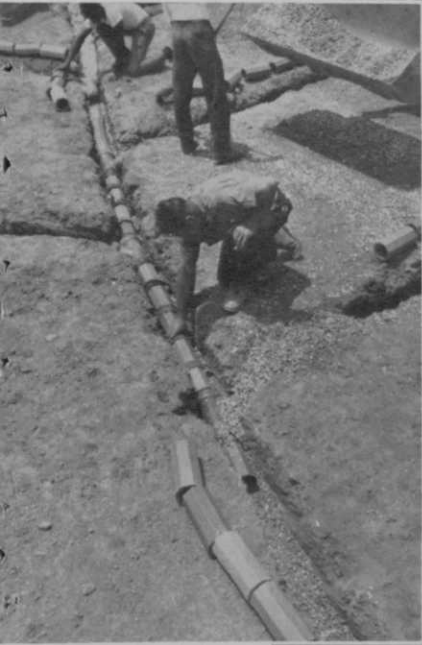
Tar paper is placed over ends of terra cotta pipe, which is laid inside the channels. Pipe is 12" long and 4" in diameter. Note T-joints of pipe where lateral trenches enter the main channel.
