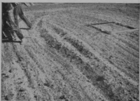
Using a drag, the treated topsoil is levelled before seeding or sodding.
