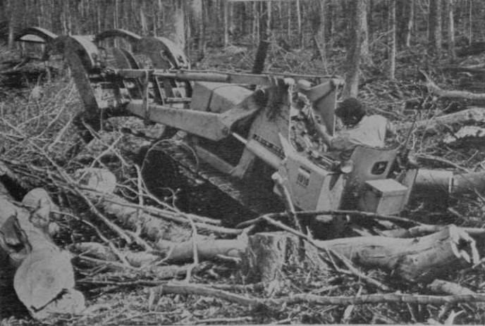
A brush and log picker smashes through heavy logs and mud in first phase of construction at the Stratton Mountain, Vt. CC. Giant claws pick up entangled trees and pile them for burning. Geoffrey Cornish designed this course.
