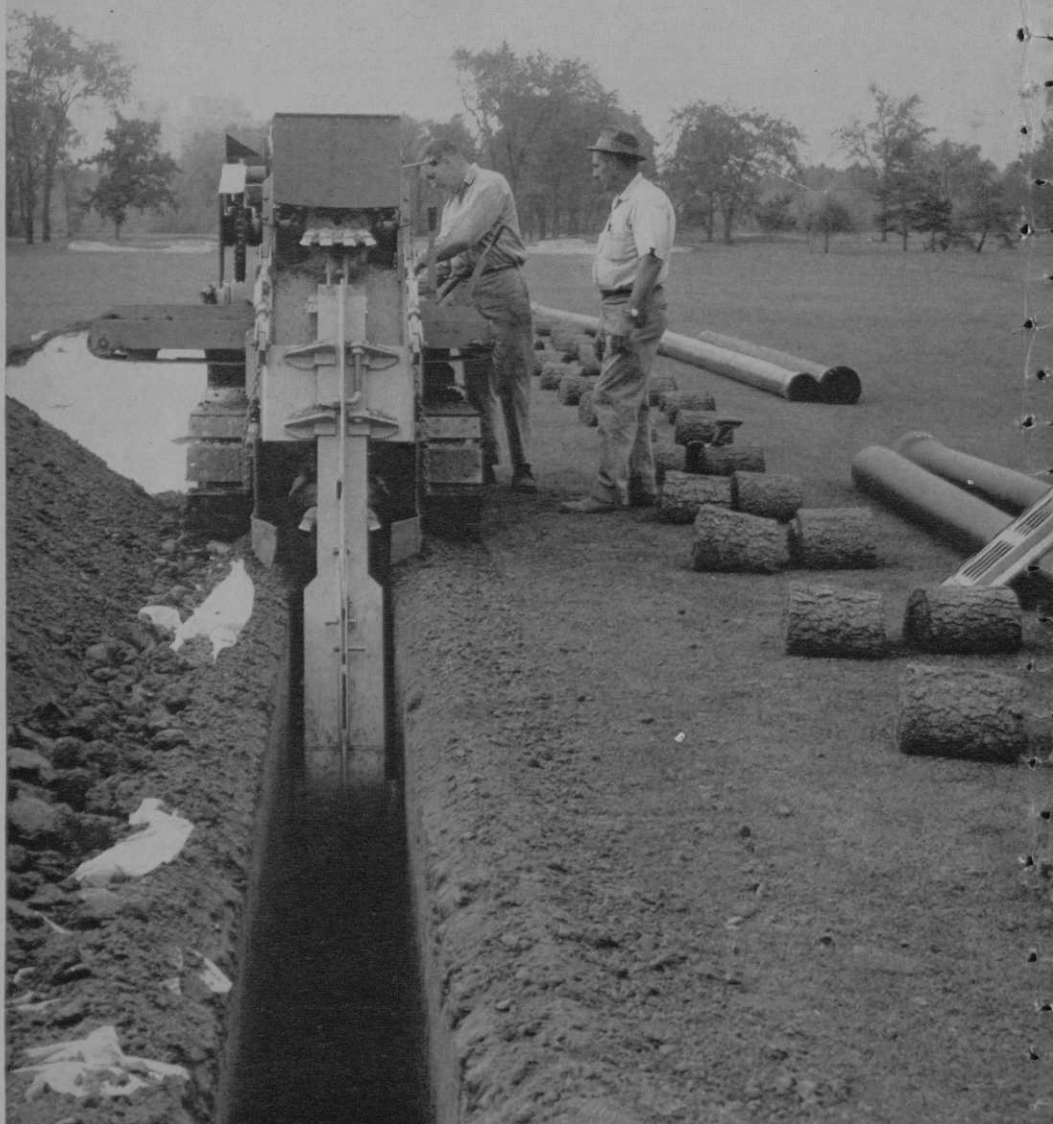
Trencher cuts a path for more than 11,000 feet of cast iron pipe used in the new irrigation system. Note plastic blanket to the left. This caught backfill and kept it from soiling the turf.
