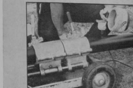
(Above) First stage in fusing Delrin pipe. Hand held heating unit is operated with power from a portable generator. (Below) Second stage in joining pipe. The pipe is ready for testing at rated pressure within 30 seconds of second stage fusion.
