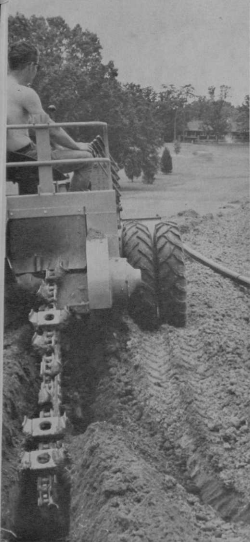
Lightweight tractor and multiple fires kept turf damage at minimum when irrigation trench was dug at El Dodaro course.
