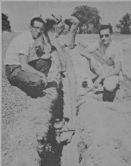
Dick Betterly, left, superintendent for the prominent irrigation specialists, A. J. Miller, Inc. of Royal Oak, Michigan, and Mark Schurman, right, inspect one of the automatic angle valves in the CRESline system.
