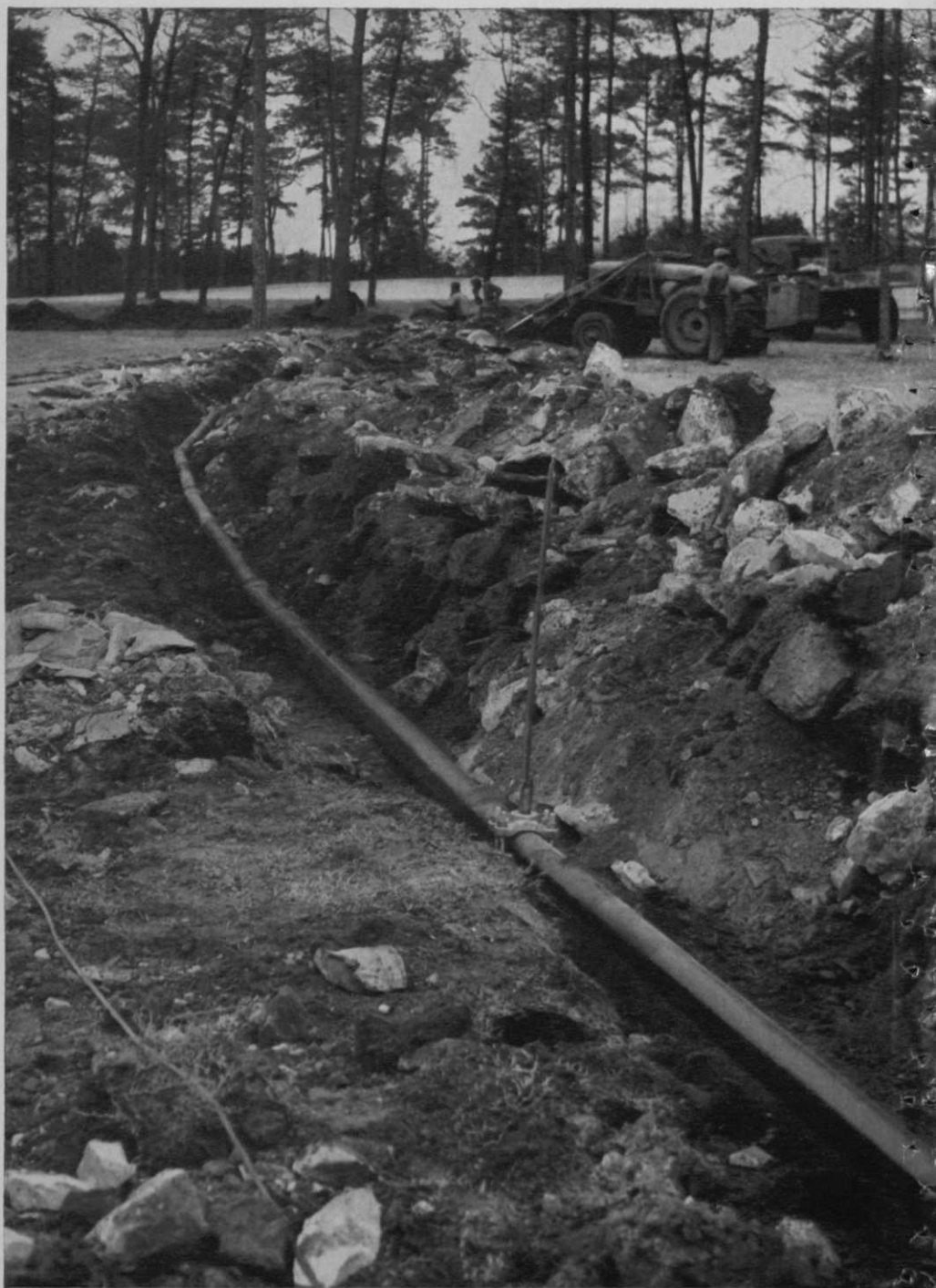
Cast iron pipe rounds a bend during extension of Vestavia's sprinkler system. Flexible joints easily adjust to rough trench conditions. No special bedding was required.
