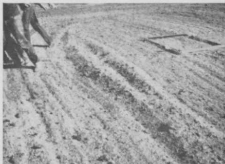
Using a drag, the treated topsoil is levelled before seeding or sodding.
