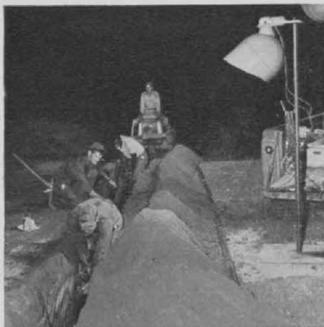
Construction crews worked nights to install a watering system on the 18-hole Broadwater Beach Hotel & GC in Biloxi, Miss. Practically all the work was done between dusk and dawn so as not to disrupt play. Entire project, including the digging of two 1,040-foot wells, was completed in 36 days.
