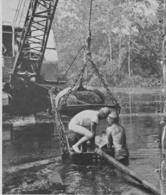
Cast iron irrigation pipe is being laid across the Mukwonago River in front of the No. 2 tee on the standard course at Rainbow Springs.
