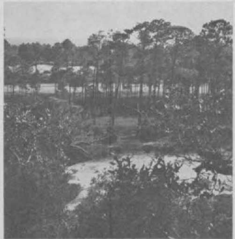
This gives you an idea of the brush that had to be cut away as Maddox crews proceeded with building of Dauphine course.
