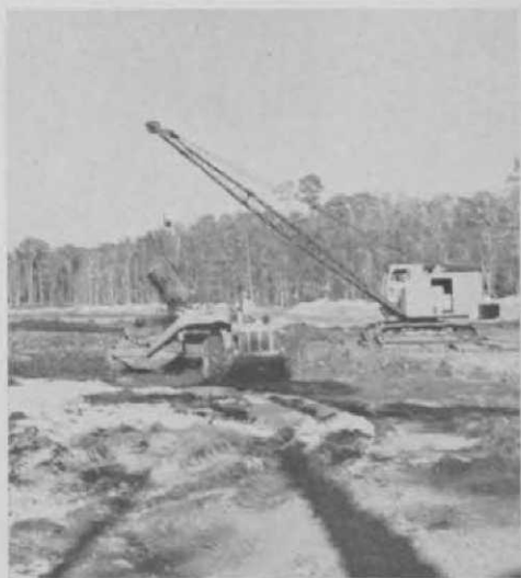
Digging silt from bottom of Alligator Lake to be used as topsoil on the course. Lake was pumped dry by Maddox firm and about 30,000 yards of silt was removed.
