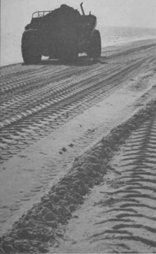
Earth mover hauls tons of silt from Alligator Lake more than one mile to Isle Dauphine course. At high tide machine often ran with one wheel in the Gulf of Mexico.
