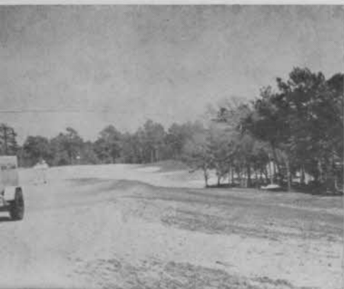
Bantam hydroseeder spreading seed, fertilizer and Turfiber on Eglin AFB (Fla.) course.
