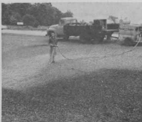
This site is getting a bath of Turfiber and asphalt emulsion for anchorage of seed in a gully.
