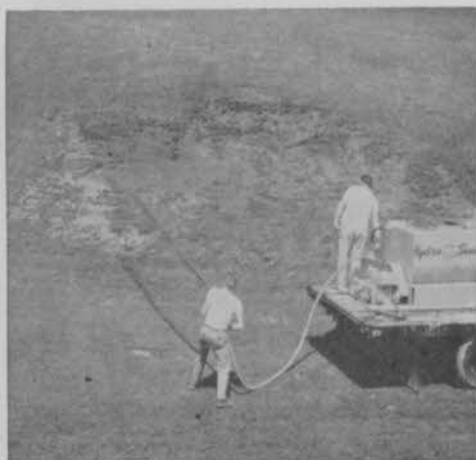
Slope on Avon Fields GC in Cincinnati is being patched with seed, fertilizer and Turfiber mixture.
