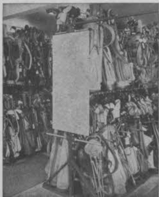
Bag Rack installation in the new pro shop of Ridge CC, Chicago.
