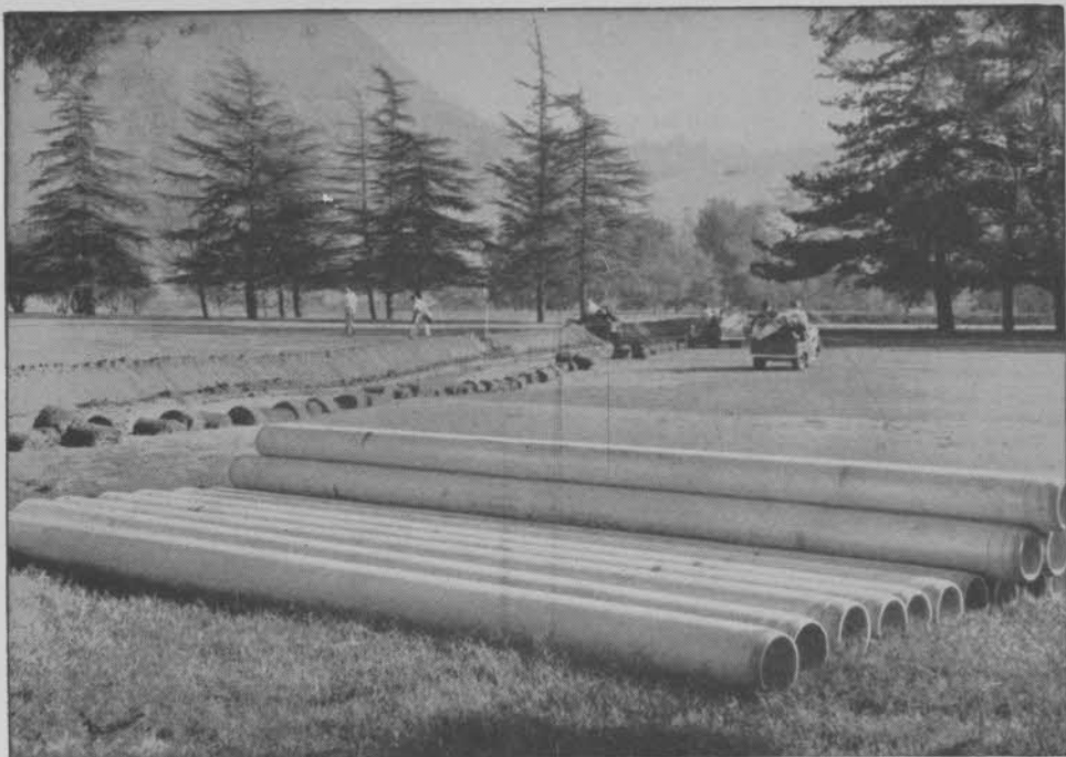
The beautiful Lakeside Golf Course, Burbank, Cal. has Transite Pipe throughout its irrigation system.
