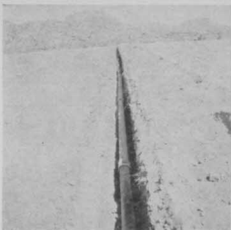
A great deal of money is spent in installing water systems to reclaim semi-arid land for golf courses.
