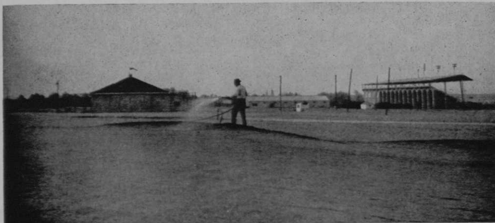
This view of the 6th green at the Woodward, Okla., municipal course, shortly after seeding, gives you an idea of the nearly impossible job of watering in a 40-mile wind, during the later stages of course building.
