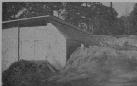
Front of soil processing building, photographed prior to finishing of road areas. The trap doors are for receiving the dumped raw soil.
