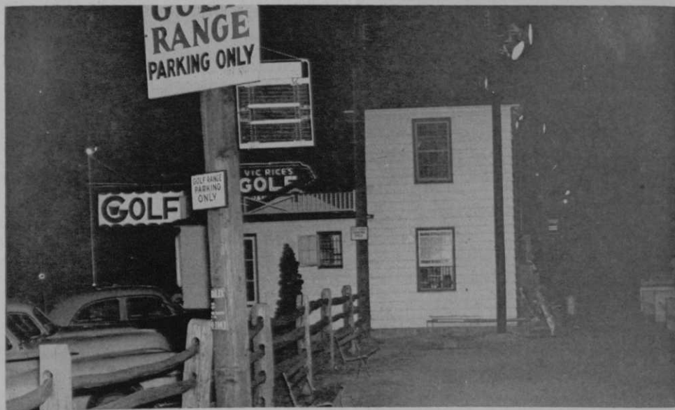
Insectocutor installed on light pole just below large parking sign at Vic Rice's Golf Range in Trenton, N. J., makes for more pleasant play by killing off bothersome insects.
