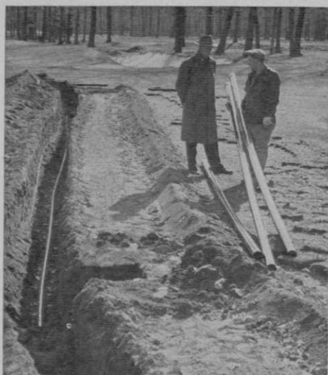
Roy S. Jones, pro, (L) and Anthony Matuza, supt., (R) inspect Triangle plastic pipe ready for installation.
