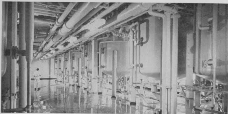
Battery of fermentors (as seen from below) used in the manufacture of antibiotics.
