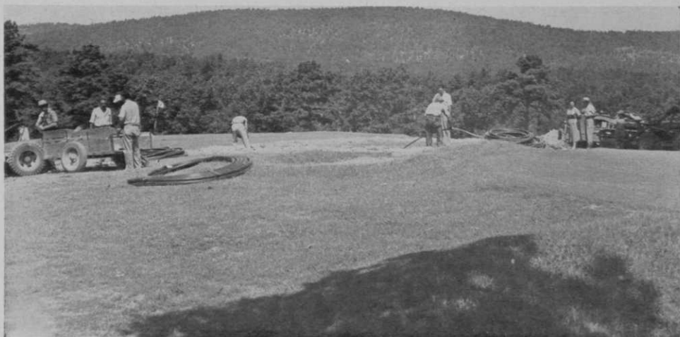
Flexibility of plastic pipe makes installation for watering system comparatively simple operation.
