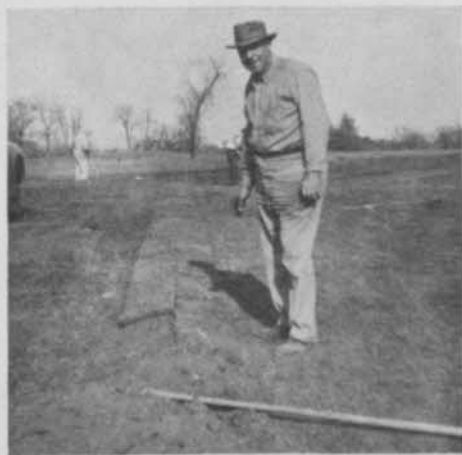
Heavy work of installing watering system was complete when ditch was filled and packed and turf relaid.
