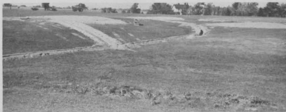
Drainage of traps around this new green (right rear) is being taken care of by tying them into the main tile system.
