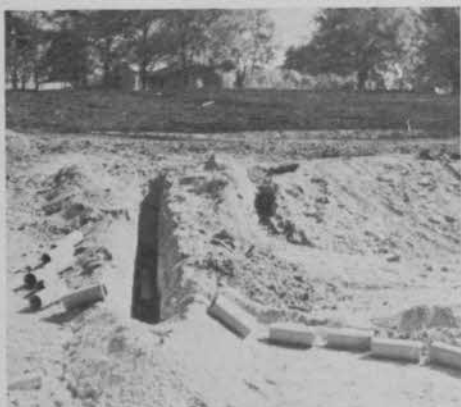
Tile was laid in the sub soil of this new green before the top soil in background was applied.
