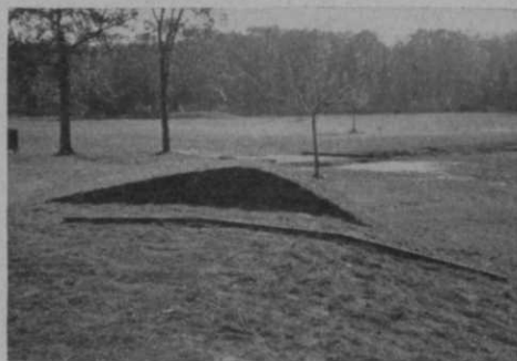
Fig. 2—Regraded bank in foreground is shown by gauge to be right for machine mowing. Compare with original grade at rear.
