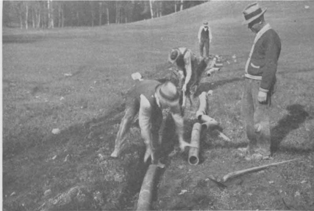
A short shallow tile line through a low wet portion of fairway costs little and helps the turf as well as playing conditions in wet seasons.
